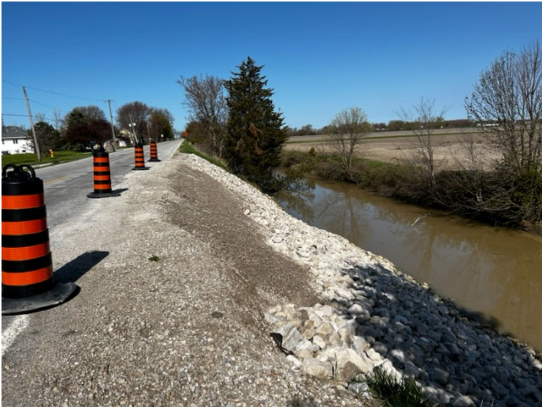
Current state of West Marsh Drain bank failure – 1424 Mersea Rd. D
