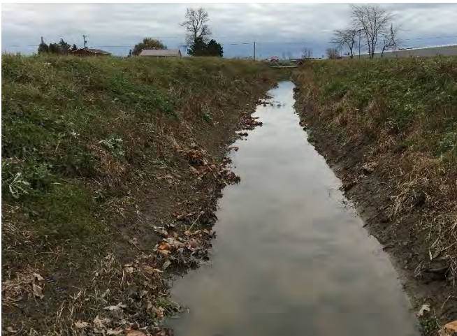
Photo 1: (SC – 7) Silver Creek Drain looking upstream towards Mersea Road 7 culvert (approximate distance 140 m).
