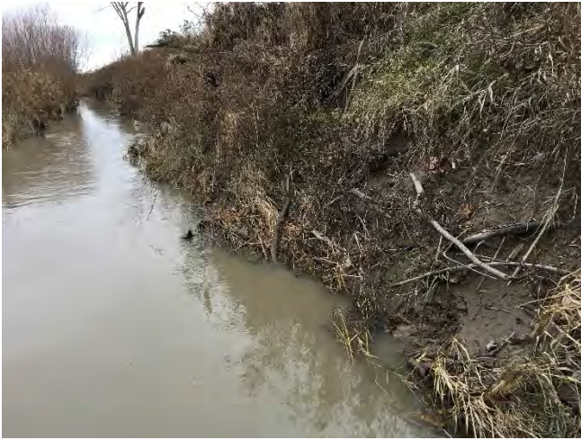
Photo 1: (SC – 8) Silver Creek Drain looking upstream, approximately 200 m North of Essex County Road 8. Some localized bank erosion is visible in the foreground.
