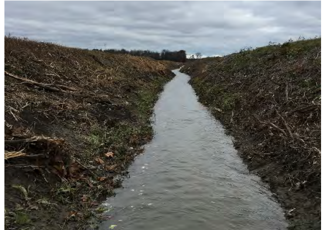
Photo 4: (SC – 14): Silver Creek Drain looking downstream approximately 100 m North of Essex County Road 14.
